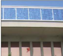
Solar Panel Array, Davis Building
