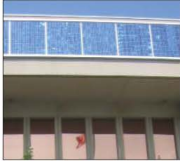
Solar Panel Array, Davis Building
