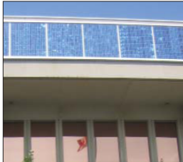
Solar Panel Array, Davis Building
