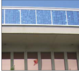
Solar Panel Array, Daws Building
