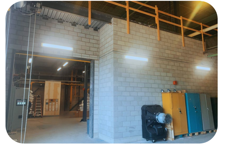
High voltage expansion room
