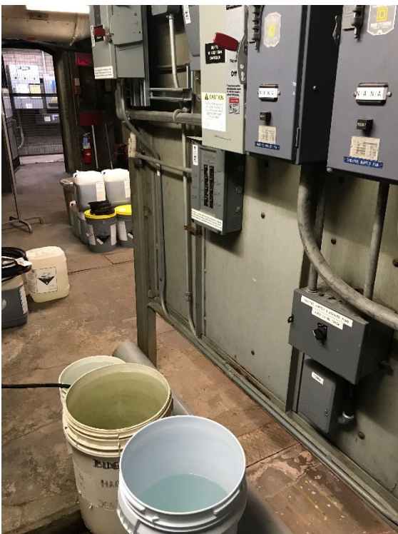
Water leaks near electrical
