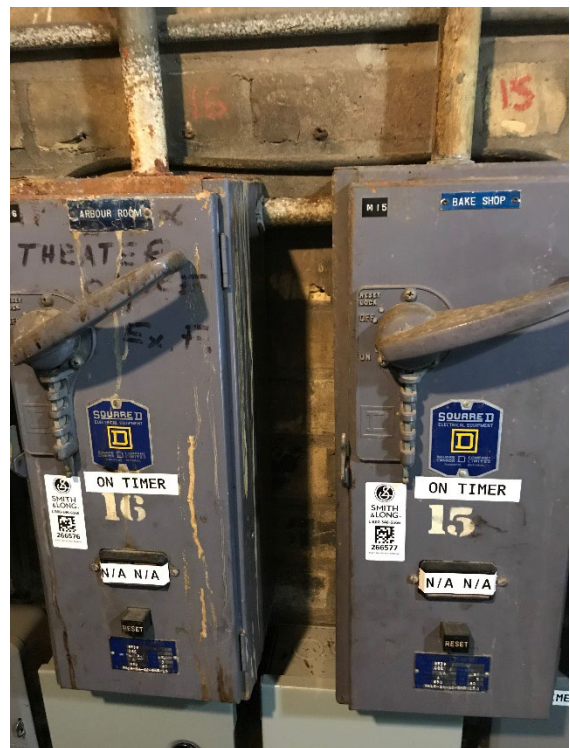
Rusting electrical components
