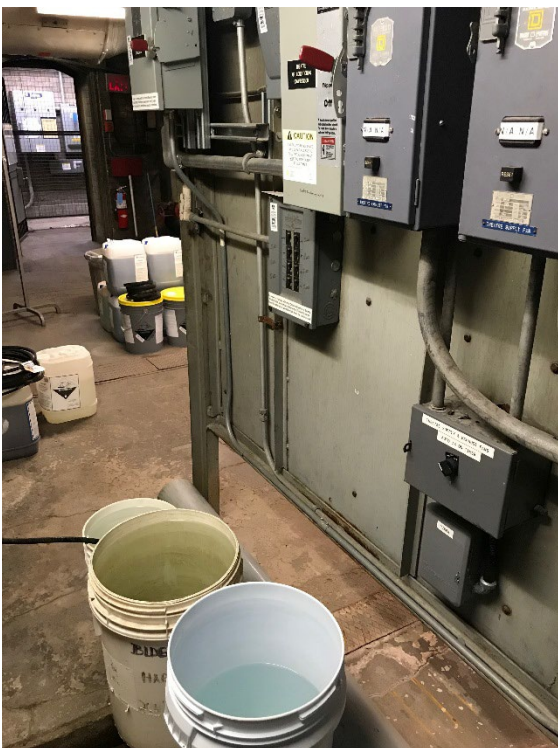
Water leaks near electrical
