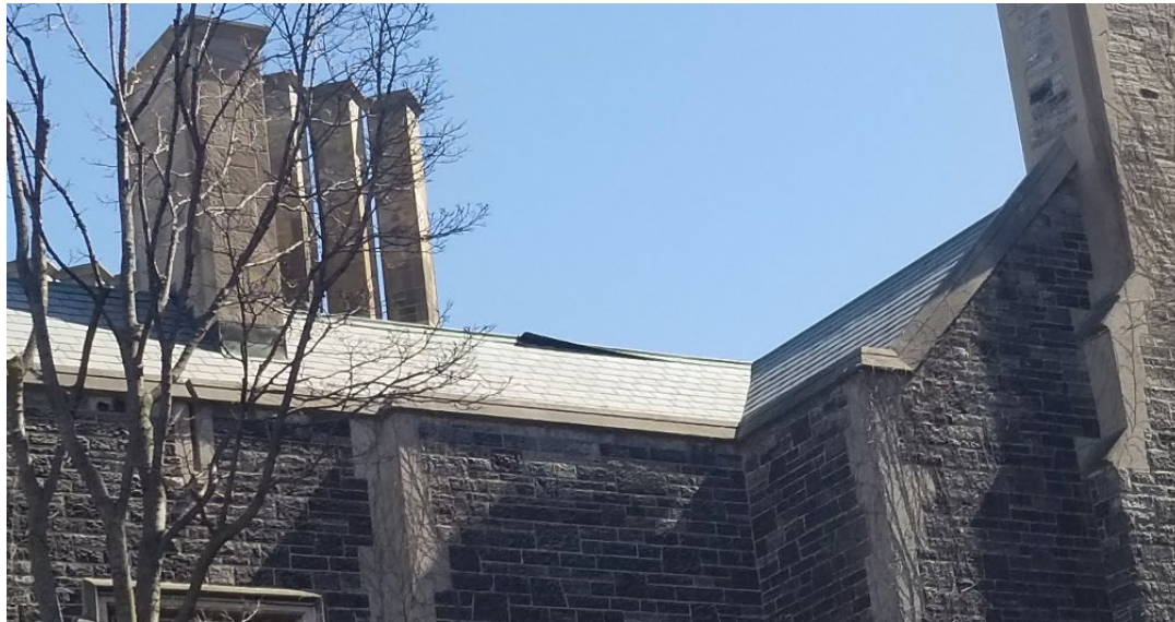
Delaminated Roof Flashing.
