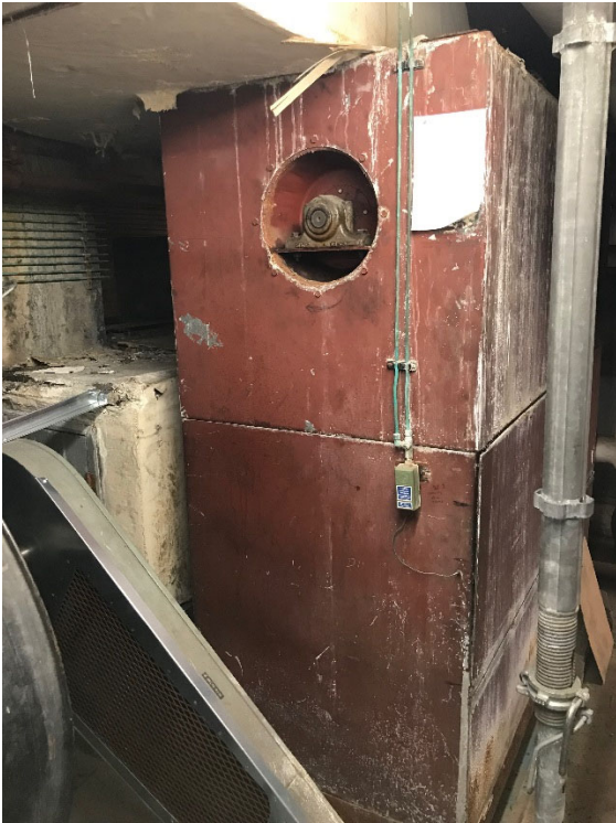
Air handler in sub-basement
