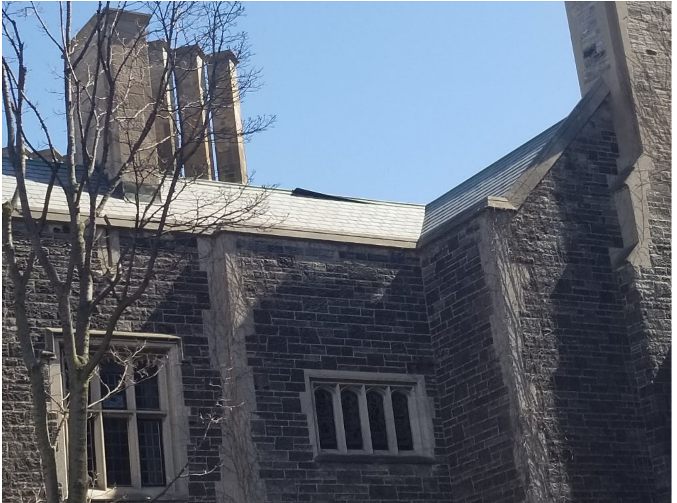
Delaminated Roof Flashing.
