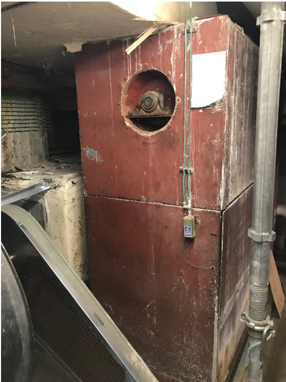
Air handler in sub-basement
