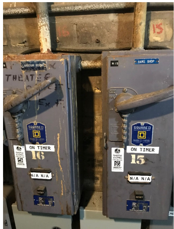
Rusting electrical components
