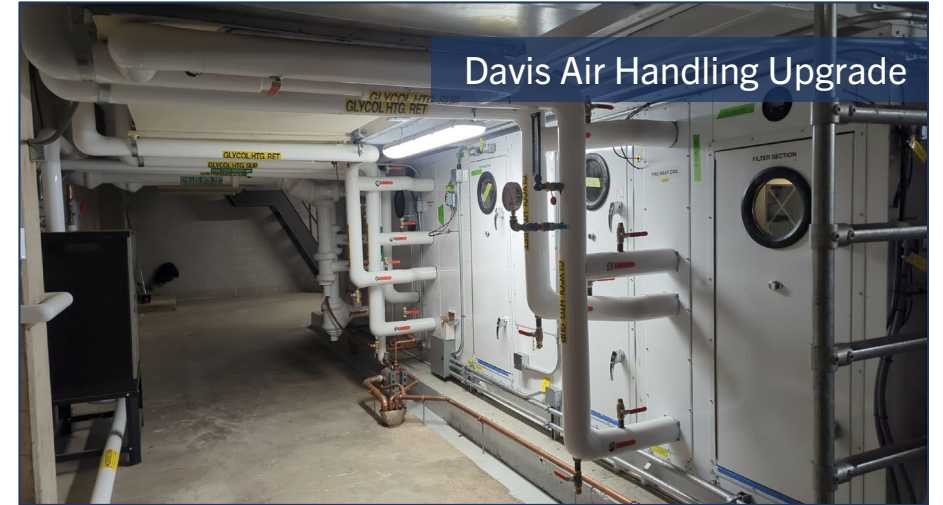
Master Services Upgrades
