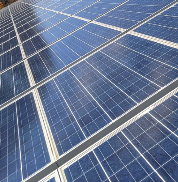
Photo: Exam Centre solar panel installation (Donglin Que)
