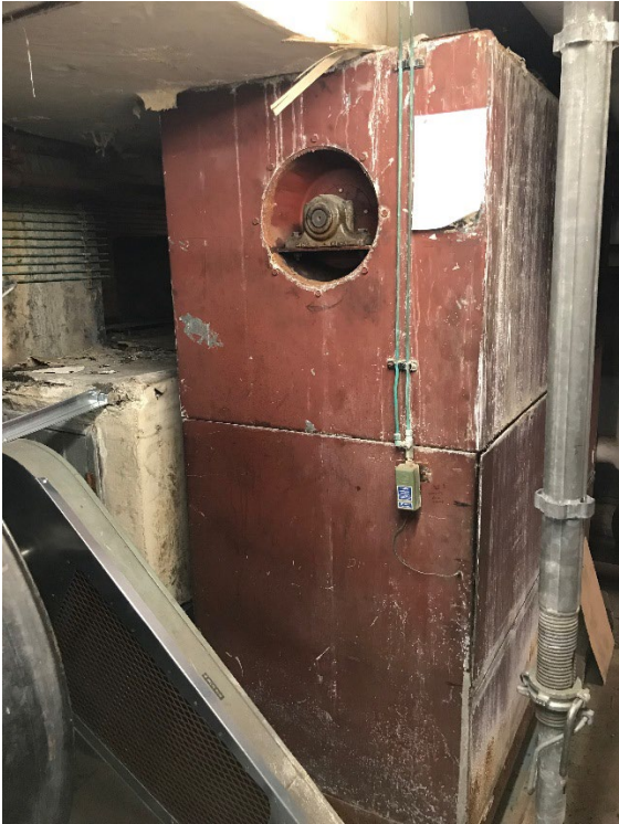
Air handler in sub-basement
