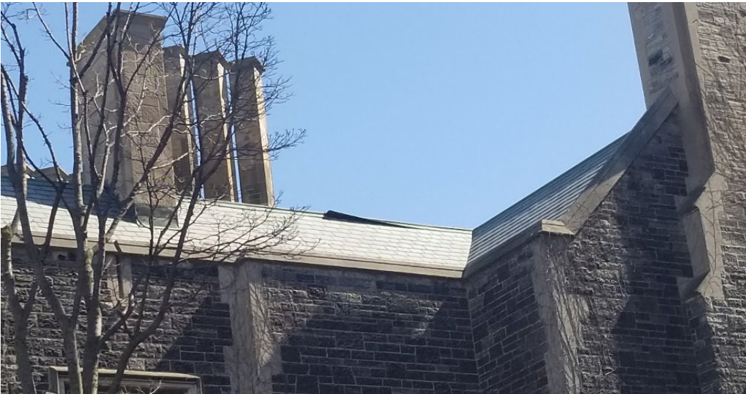
Delaminated Roof Flashing.
