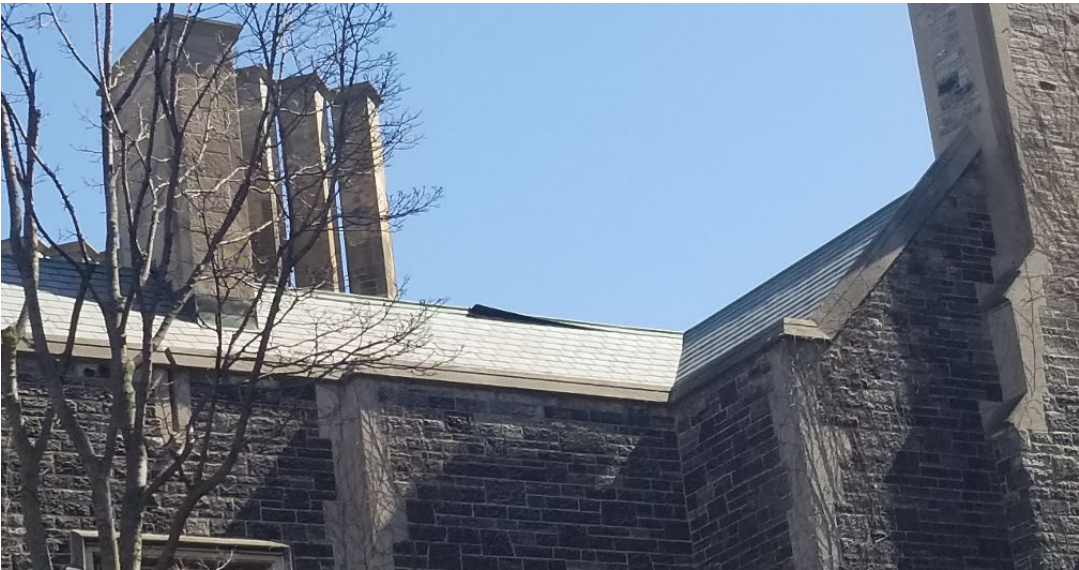
Delaminated Roof Flashing.
