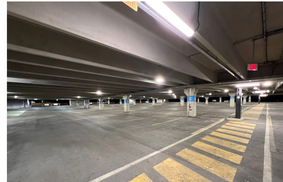
New LED P8 Parking lighting
