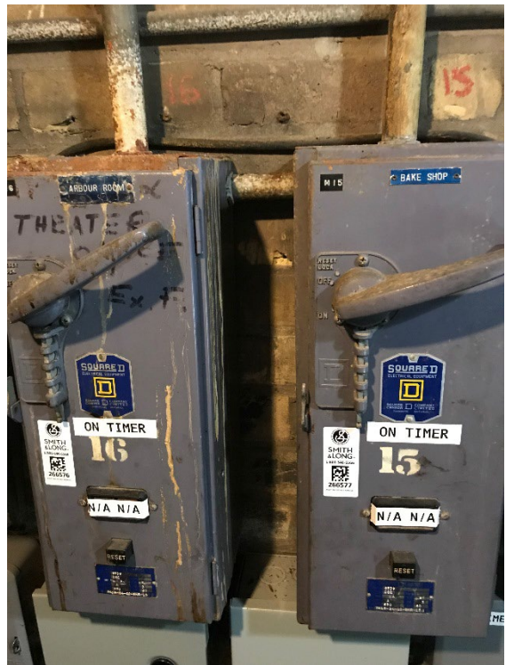
Rusting electrical components
