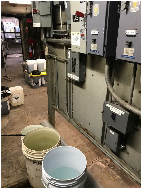
Water leaks near electrical
