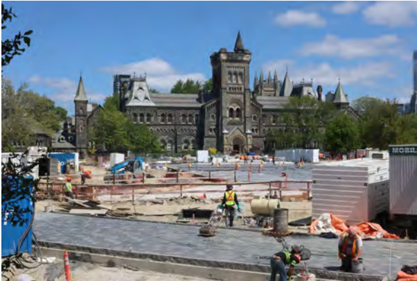
Before: Construction of Canada's largest urban geothermal exchange. Photo by David Lee.
