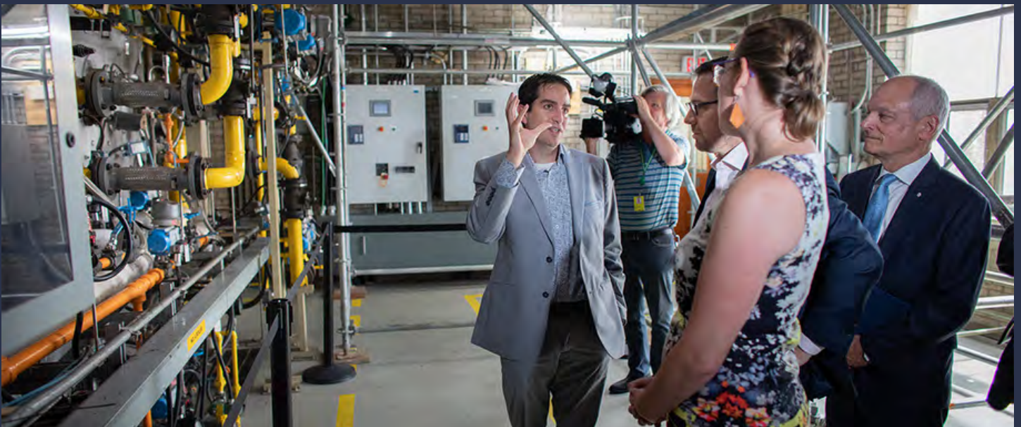
Ron Saporta, U of T's Chief Operating Officer, Property Services and Sustainability and CECCS Co Chair, shows Karina Gould, families, children and social development, President Meric Gertler, and Ehren Cory, CEO of CIB, the Landmark Geothermal project currently under construction. (Photo credit: Johnny Guatto.)
