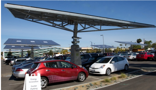
Roof-mounted photovoltaic panel example
