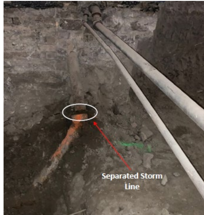
Damaged piping beneath the Arbor Room
