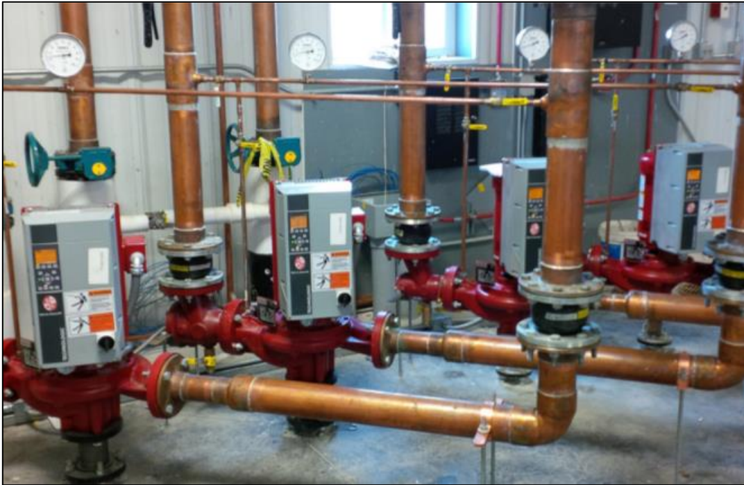
Figure 21 – Site Distribution Pumps
