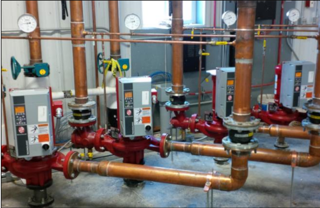
Figure 21 – Site Distribution Pumps
