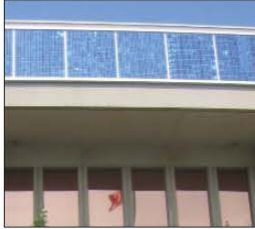
Solar Panel Array, Davis Building
