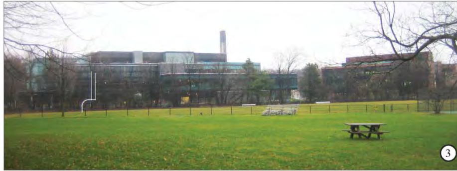
View of athletic field (future Campus Green) and Instructional Centre under construction
