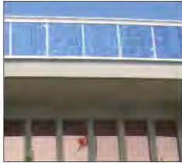
Solar Panel Array, Davis Building
