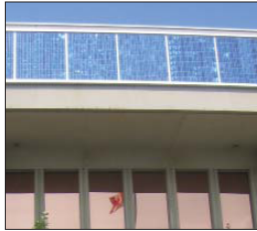
Solar Panel Array, DAVIS Building
