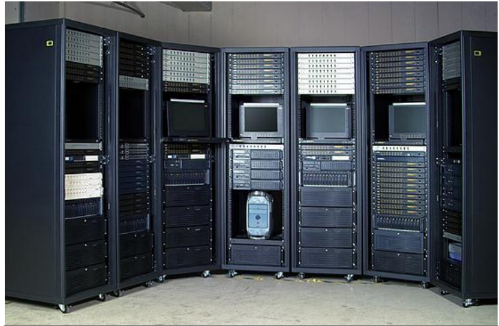
Figure 17. Example of server storage.
