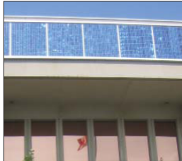
Solar Panel Array, Davis Building
